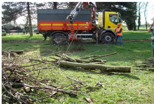
Figure 5. Tree felling in Lombardy, Italy for citrus longhorn beetle control. ©Neil Giltrap and Dominic Eyre, Defra
